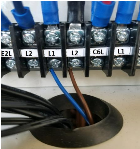
Pump POWER wires.
